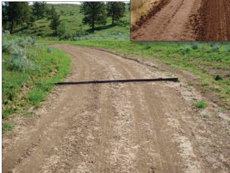
► Above & left: These photos show improved roads with rubber water diverters installed to reduce erosion.
