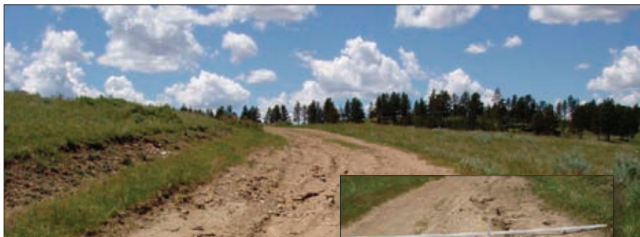
► Above & right: These photos show eroded gullies on pasture roads.
