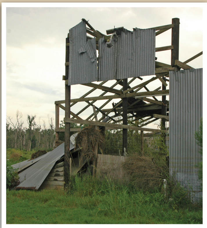
► Right: Pomes' horse barn is in ruins after Hurricane Katrina filled it with 8 feet of water.
