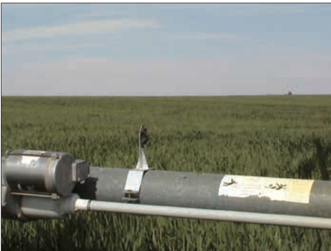
►A wire clamp with an insulator is fixed to the tower brace pipe and works to stabilize the wire by keeping the wire from grounding on the pipe or on the drive motor.
