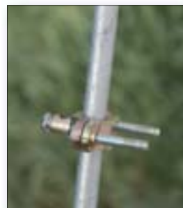
► For an effective ground, the ground wire should be securely fastened to the ground rod with a brass or stainless steel clamp.
