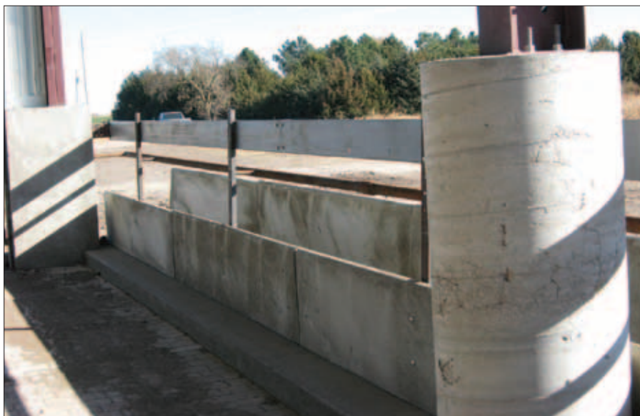
►Poured concrete bunks feature a step — about 10 in. wide and 6 in. high — to aid young calves in reaching feed. The step also helps prevent cattle from backing up to bunks and defecating inside.
