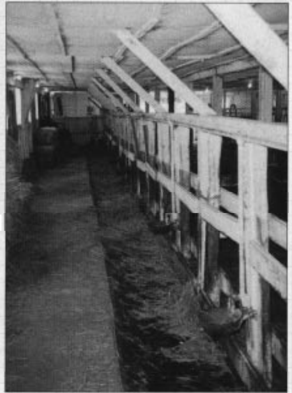
(Above) A view of the barn's east side center alley and cement feed mangers covered with plastic liner.
