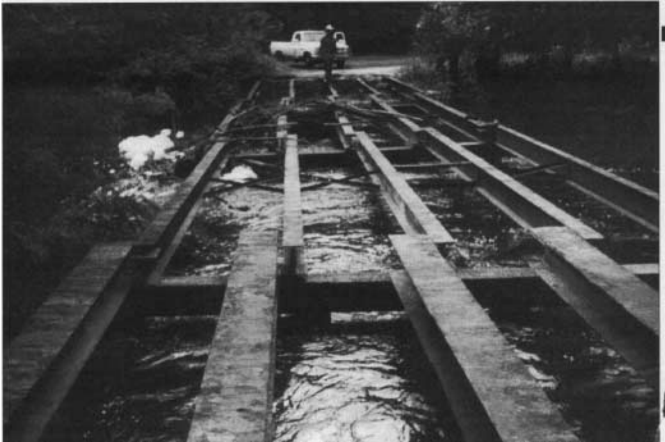
Remains of a bridge across a creek on Lane Holton's farm near Camilla, GA.
