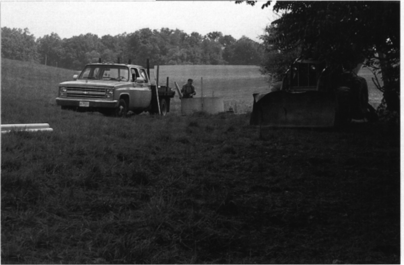
Installing spring watering tanks in each pasture provides clean fresh water for the McGinnis herd.
