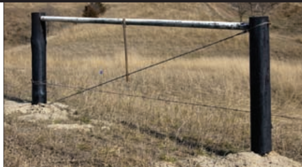
►Part of new fence going up on the Haumont Ranch near Broken Bow, Neb., this "H-brace" is constructed of 8-in. posts (8 ft. long) set 4 ft. into the ground. The horizontal brace piece is an 8-ft. length of 3½-in. salvaged pipe. The diagonal brace wire is 9-gauge galvanized wire wrapped twice around the posts and twisted tight with a "twitch."
