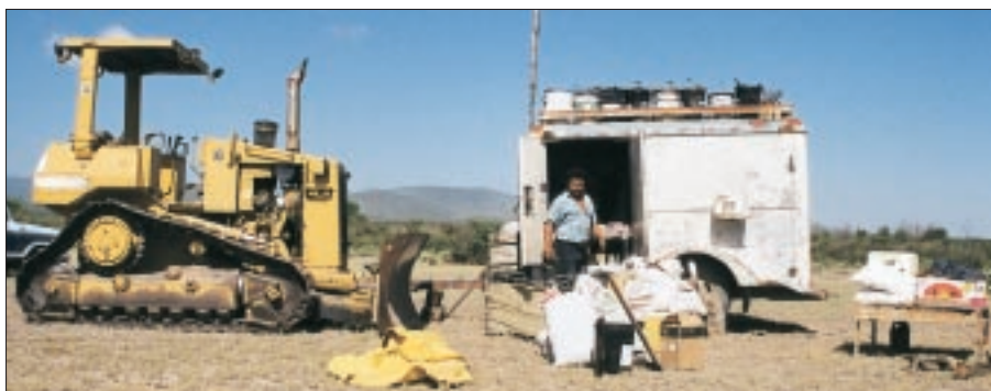
Carlos and Juan spent each day building dirt tanks, or ponds, across this arid ranch. The white trailer was towed behind the dozer between digging jobs. It came complete with cots and "girly calendars" for these heavy-equipment operators. All cooking was obviously done over an open fire.
